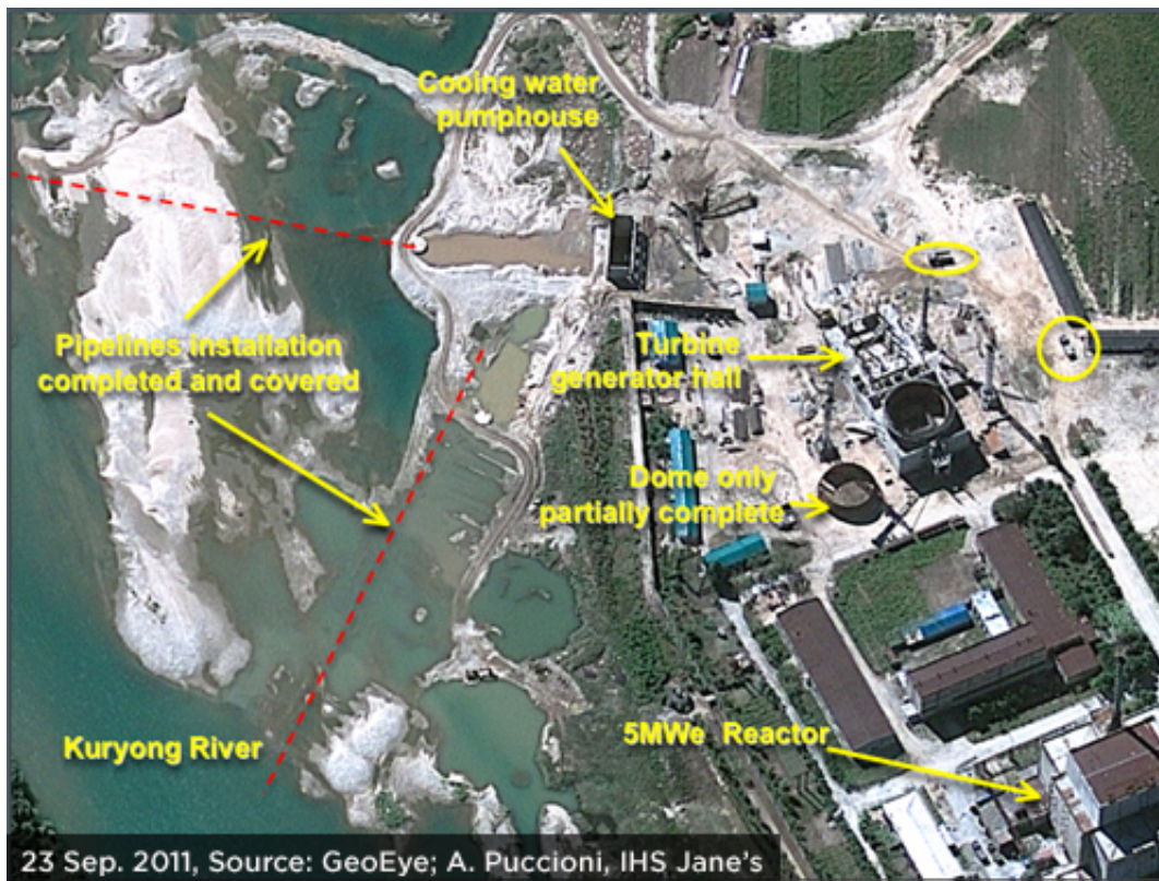
Annotated diagram of the new reactor site, shown in a photo indicating significant progress in construction.
